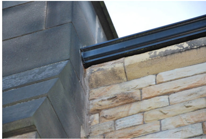
Typical gaps in masonry
