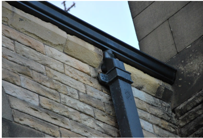
Typical gaps in masonry
