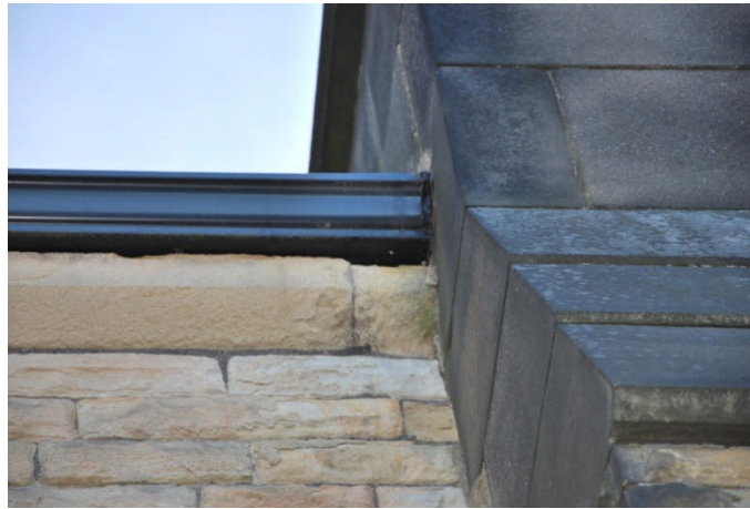
Typical gaps in masonry
