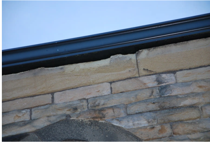
Typical gaps in masonry
